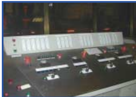
Main Control Pulpit
