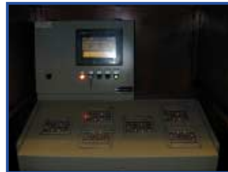
Local Control Panel
