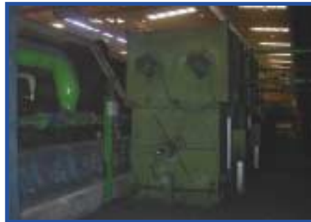
DC Motors Mill Stands
