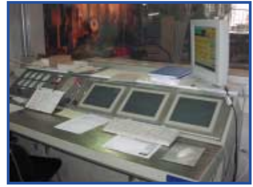
Main Control Desk
