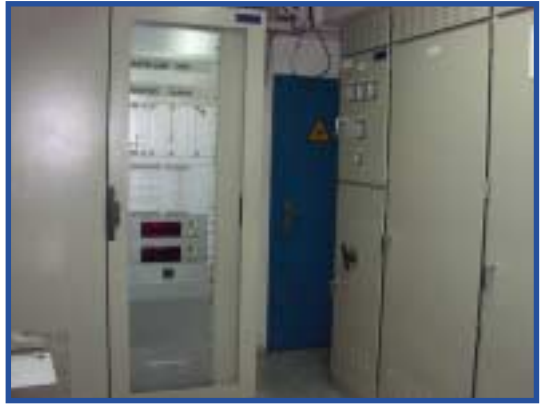
Auxiliary drives and Electrodes Control Equipment
