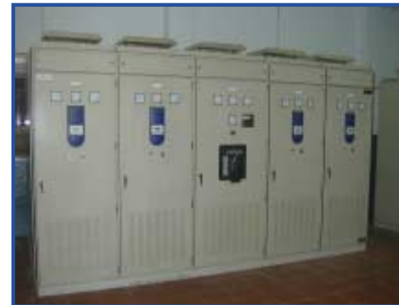
DC Motor Control Center
