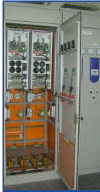
Auxiliary VVVF Cabinet
